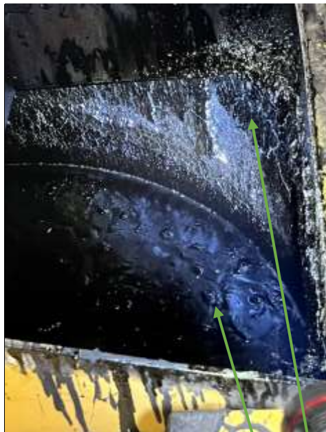
FLAKES IN MATERIAL FROM BUILDUP
